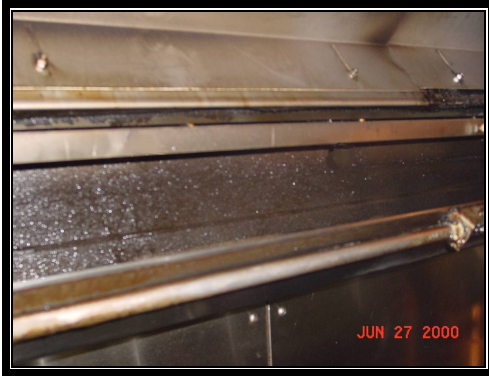
Inspect Baffle Positions
